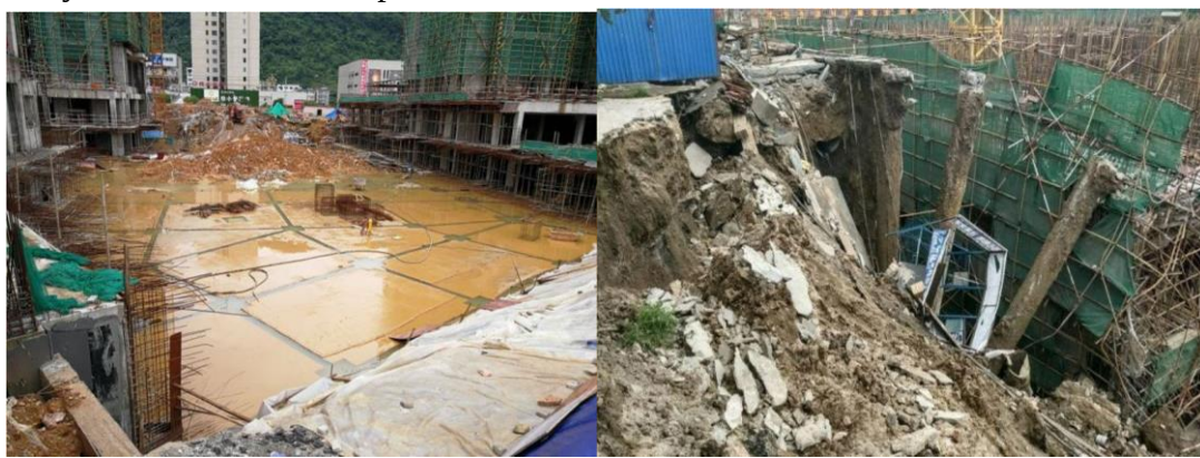
Figure 4 A "mess" pattern of construction
